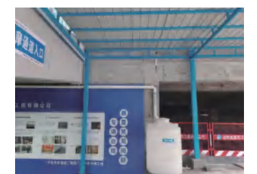
Rainwater Collection Tank
